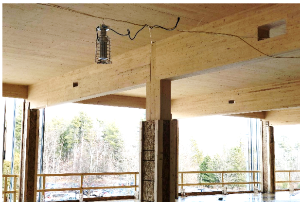
Figure 13: Beam-to-column connection. Column width is notched down to allow direct beam bearing. 90 Arboretum Drive Office Building, Newington, NH. Source: WoodWorks
