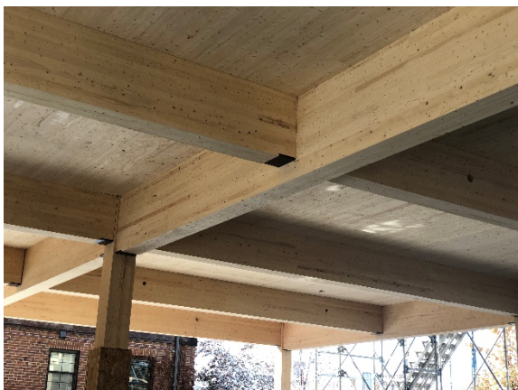
Figure 3: 24x24-ft grid at Denver University’s Burwell Center for Career Achievement. Source: WoodWorks
