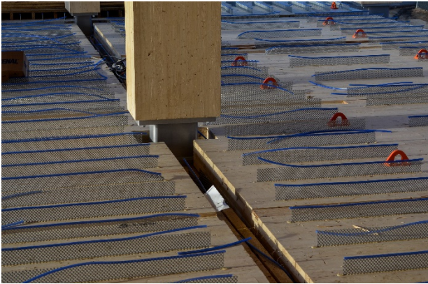
Figure 9: John W. Olver Design Building, University of Massachusetts, Amherst, MA. Shear connectors for CLT-concrete composite installed in top of CLT prior to concrete placement. Source: Alexander Schreyer
