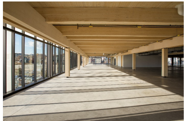
Figure 4: Platte Fifteen, Denver, CO. 30x30-ft grid with two intermediate beams and 3-ply CLT. Source: Oz Architecture, KL&A Engineers & Builders, photo JC Buck
