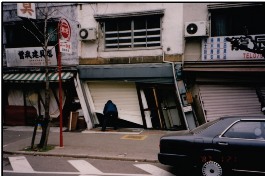
Figure 2-13 Severe leaning and incipient collapse of a two-story mixed-use building in Kobe City.
