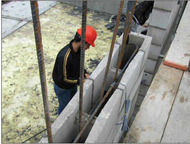
Figure 7-3. Anchorage of horizontal bars around vertical bars with a standard hook in a horizontal plane.
