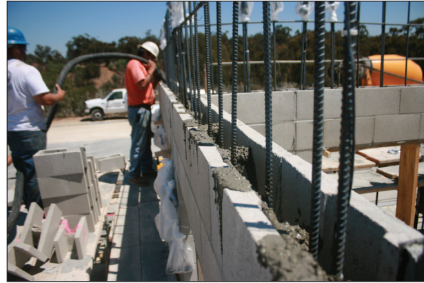
Figure 7-2. Grout flow is facilitated in a fully grouted wall with open-end masonry units.
