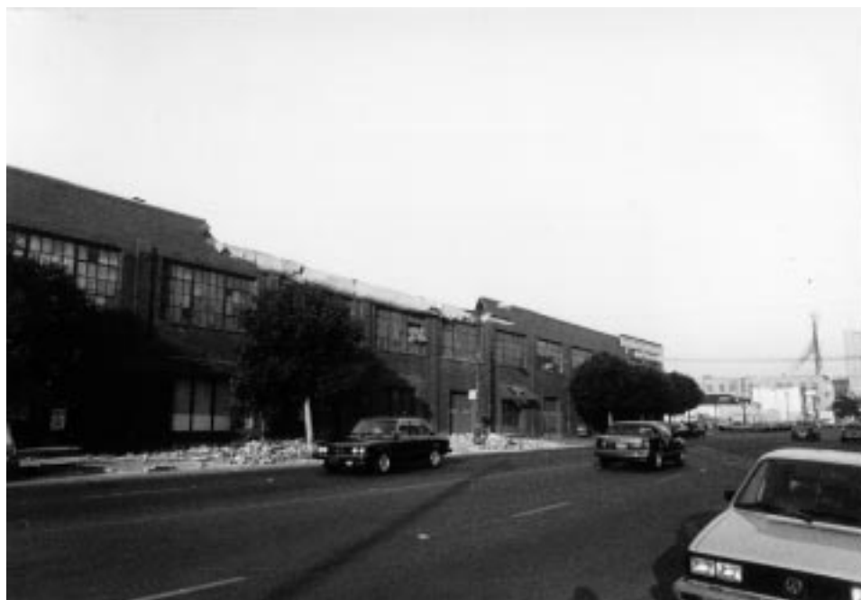
Figure 7-2 Photo of Parapet Failure (from Rutherford and Chekene, 1990).
