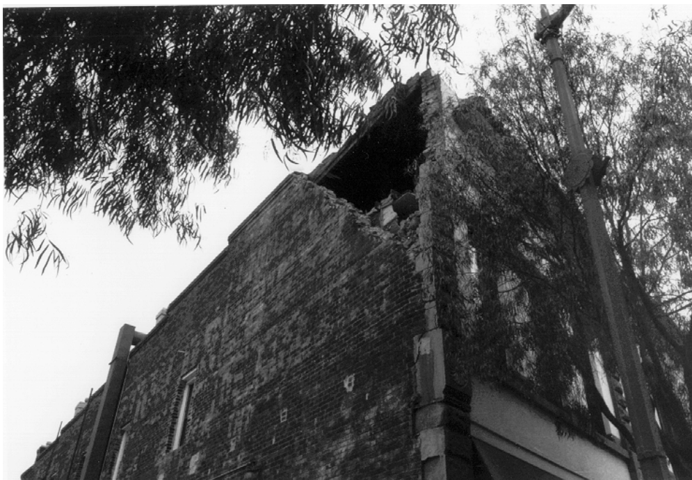
Figure 7-12 Photo of Corner Damage (from Rutherford and Chekene, 1990)
