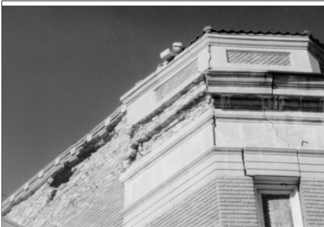
1994 Northridge Earthquake: Santa Monica.
